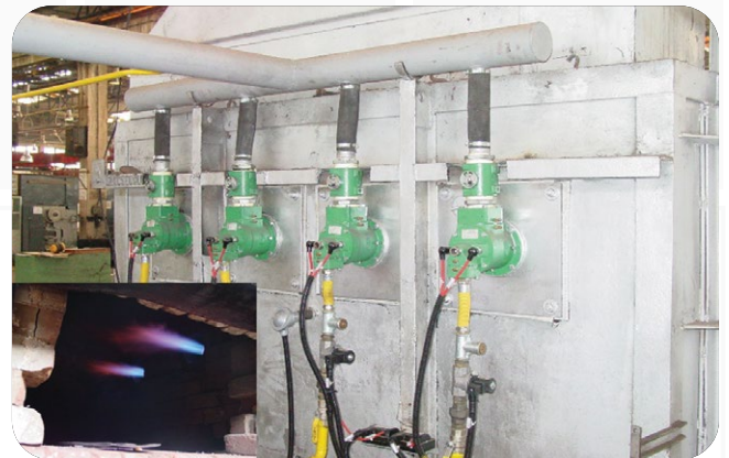
Product : Industrial Process Burners Application: Conditioning Furnace Burning System
