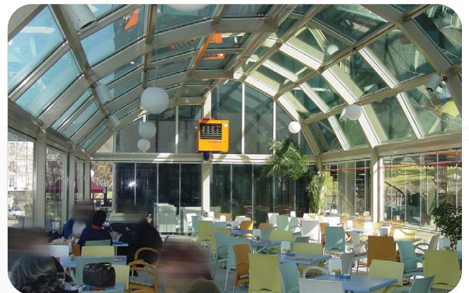
Product : Warm Air Heaters Application: Café Ambient Heating
