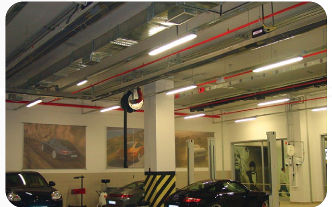
Product : Tubular Radiant Heaters Application: Car Service Station Ambient Heating
