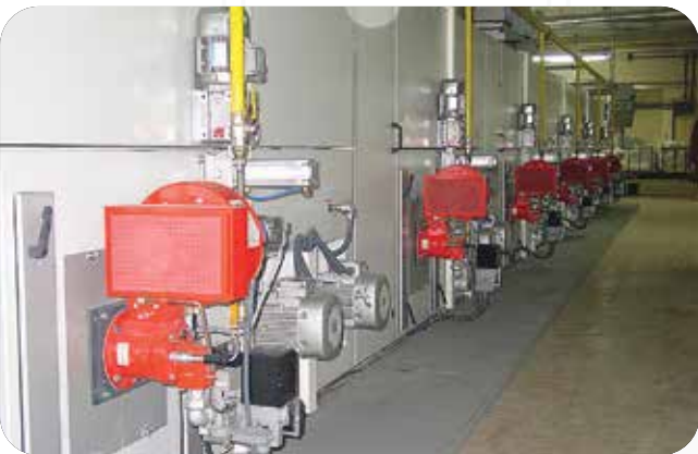
Product : Industrial Process Burners Application: Stenter Machine
