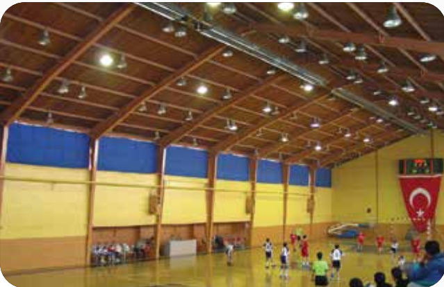
Product : Tubular Radiant Heaters Application: Sports Hall Heating
